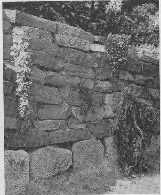
On this wall of stone slabs a few trailing plants make it interesting without altering its character.
