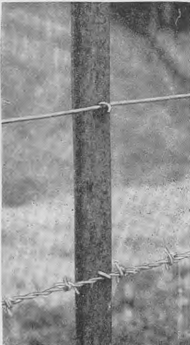
Staples are used to hold the wires to an H-section steel post driven into the ground.
