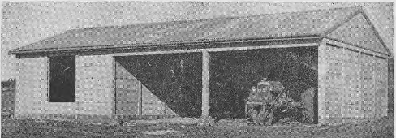
Buildings should be constructed with materials which will give greatest permanence with least maintenance. This implement and storage shed was built of foamed concrete units by 4 men in 8 days on a site 230 miles from the factory supplying the units. The cost was 10s. per square foot.
