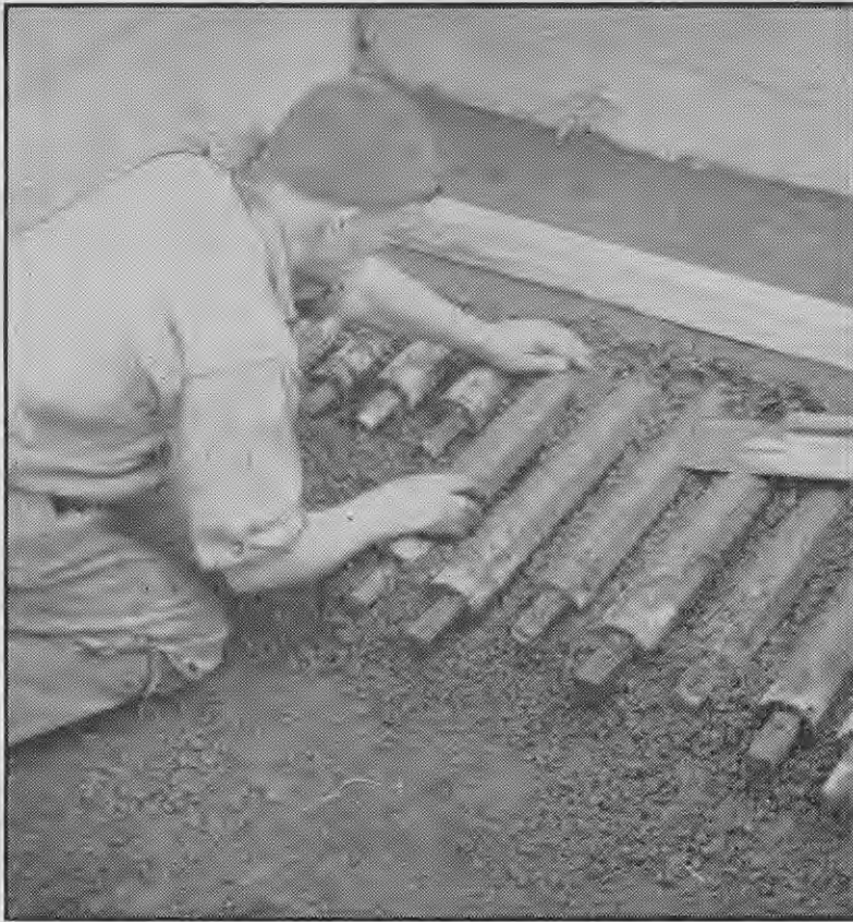
["New Zealand Farmer" Laying coke breeze (shown above) or other well-insulated sleeping floors will pay good dividends.
