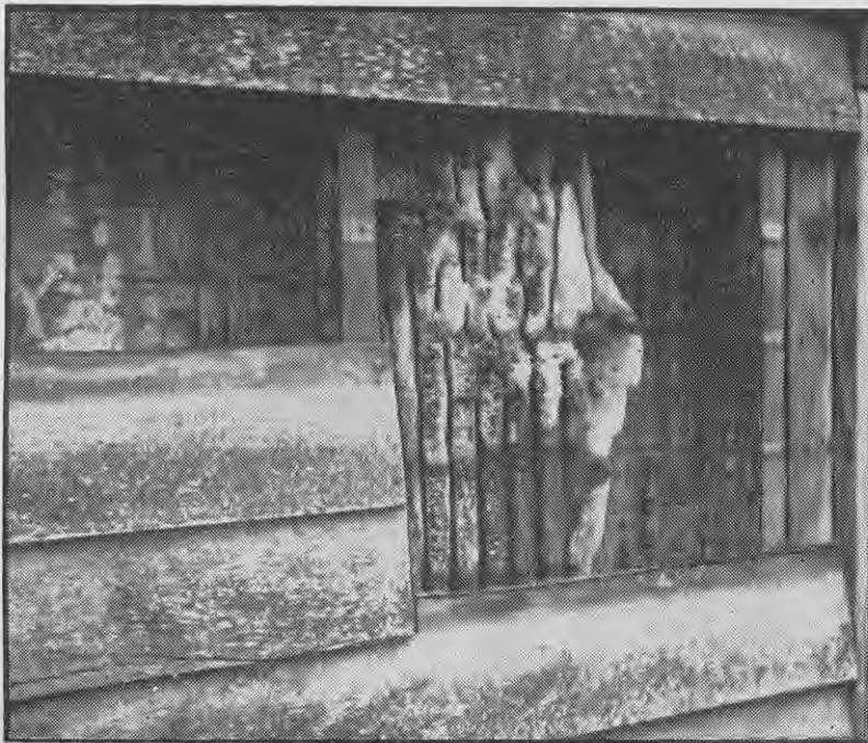
When this farm building was opened up the bees were found to be diseased.
