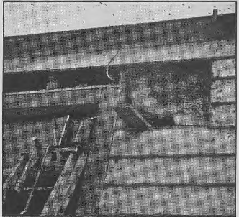
Wall opened up. The old comb is examined for disease before the bees are destroyed.
