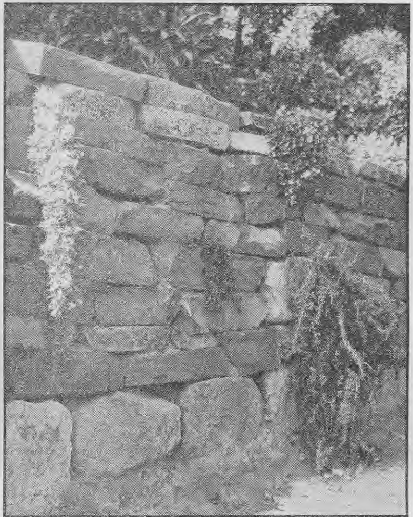
[V. O. Brown] A stone retaining wall with trailing plants in bloom. The foundation stones should be sunk at least 10in. into the ground and placed on a solid rammed foundation. This wall was built with very little forethought for the needs of plants growing on its surface. The stone should be sandwiched with 1 to 3in. of soil packed into position. The interstices between the stones may be 2 to 4in., being larger between big stones. Plants are set in soil packed between the stones. In spite of certain faults in construction of this wall, trailing campanulas are making a brave show on it and Rosmarinus officinalis prostrata appears to be thriving.
