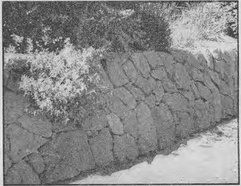
F. C. Browne A stone retaining wall with each stone fitted with its neighbour. A good feature is the large stones at the base and the smaller ones at the top. The interstices between the stones prevent the build-up of pressure of the weight of moisture and sodden soil in wet weather. If this wall were to be used for growing plants, the stones would be better trimmed and built horizontally, 1 to 3 in. of soil placed between them, and the stones bonded. Drainage behind, through, and at the foot of the wall is also required and is essential in wet districts. Coverage of the wall as it is would best be achieved by insertion of trailing plants at the top and small shrubs and climbers at the base; in 2 or 3 years very little of the wall would be visible.
