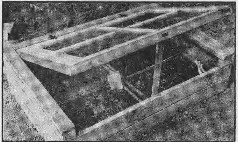
[E. W. Orr A window sash is useful as a frame top, but as it does not shed water, the woodwork is likely to rot fairly quickly.
