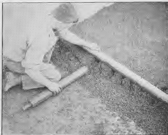
The final section completed, the mandrels are completely withdrawn and the ends of the cavities sealed with another layer of the mix.
