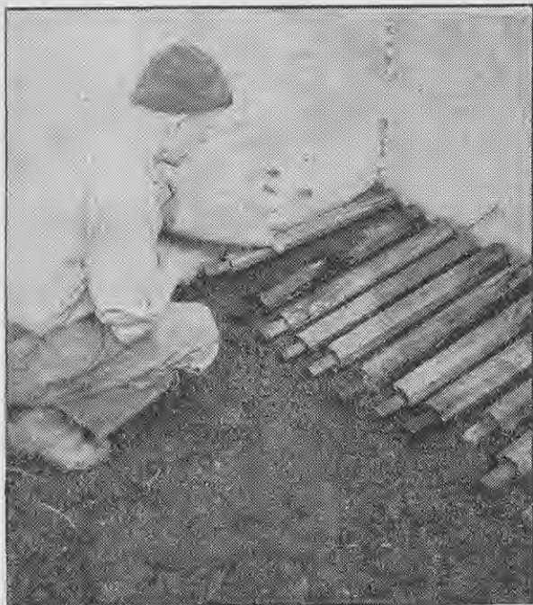
Mandrels laid in position for the first section of the floor. The bedding layer of breeze concrete has been brought clear of the fronts of the mandrels.
