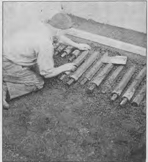
Another bedding layer of mix is put down and the mandrels carefully drawn out on to it. Note the position of the left hand to prevent disturbance to the concrete previously laid.
