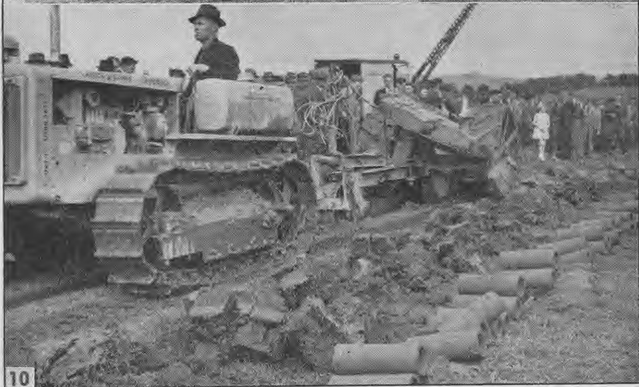
9. The Lewis digger making the second run. Another drain is cut on the return run to the beginning of the first; this puts the spoil all on one side of each drain. 10. The Lewis digger in the second cut; 3 or 4 cuts are required for each drain 24in. to 26in. deep. (Note: By fitting larger discs greater depths can be obtained; likewise the width of cut can be reduced or enlarged by altering the space between the discs.)
