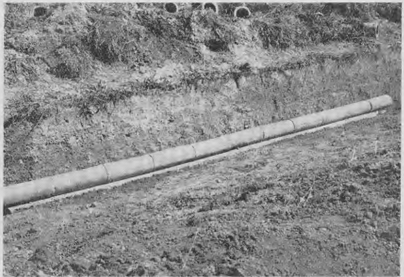
Where the tiles have to be laid over a soft area a board may be placed underneath to prevent subsidence.
