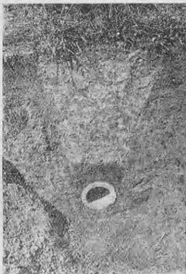
A cross-section of a well-finished pipe drain. The bottom of the drain was little wider than the tile, and movement is consequently impossible.
