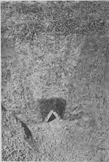
Another type of slab drain popular in the early days of abundant timber supplies.
