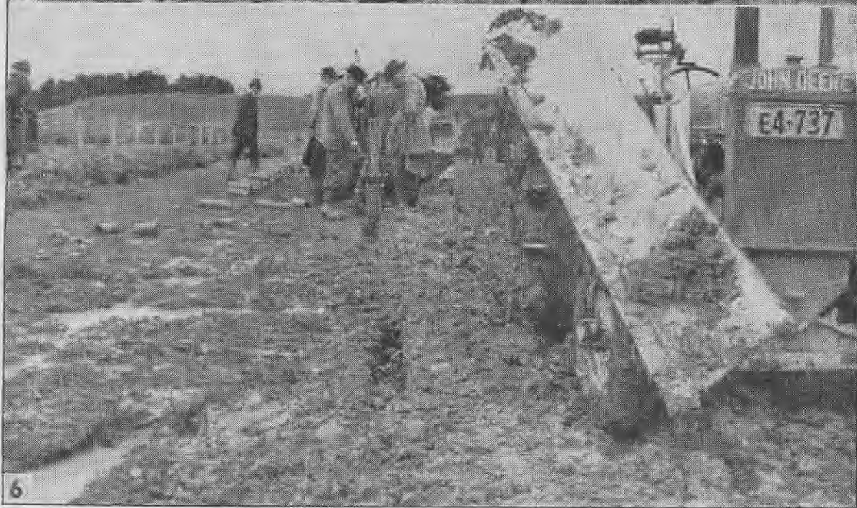
5. The angle dozer backfilling. With all spoil to one side as left by the "Rotohoe," one run of the machine will do the job. 6. The angle dozer blade lifted to the carrying position.
