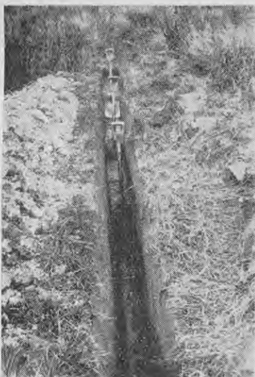
An ordinary spade leaves the bottom of the drain too wide and displacements will follow. The last spit should be removed with a draining spade and the bottom cleaned with a draining scoop.
