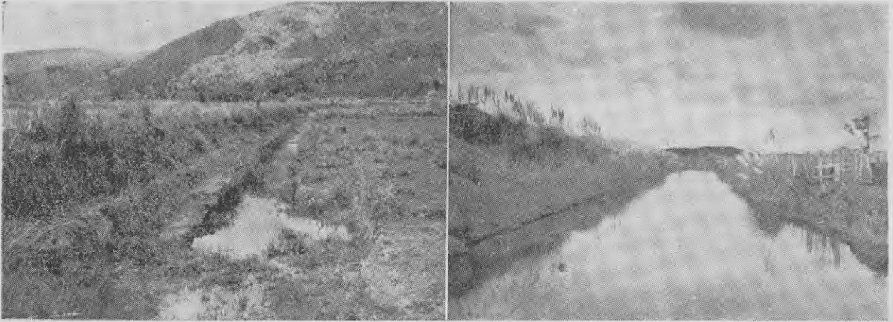
Left—A stopbank of considerable age showing main drain inside bank and step between edge of drain and stopbank. Note strong protective growth of buffalo grass on bank. Right—Large stopbank and drain on large reclamation. Stopbank has been constructed with material from drain by means of a grab dredge. Note protective covering of strong growth of buffalo grass and pampas grass on stopbank.
