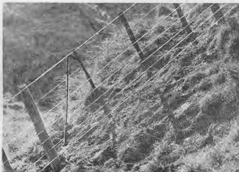
Fig. 14—How posts and battens should be placed on a steep hill face. The line of the string suspending the hammer shows the perpendicular.
