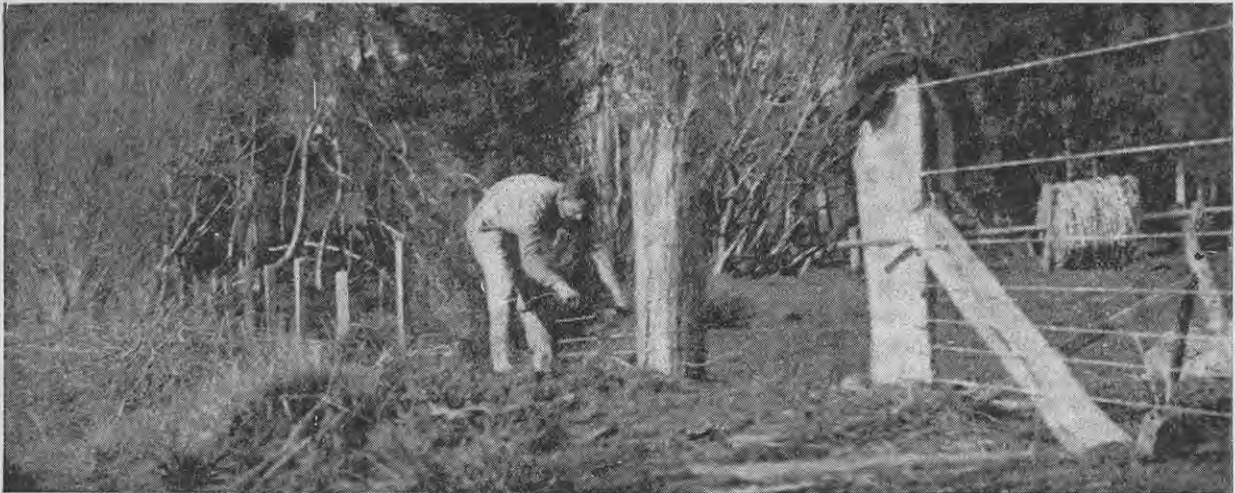
An experienced group workman is competent to tackle any kind of farm work from scrub cutting, draining, or concreting to relieving in the milking shed.
