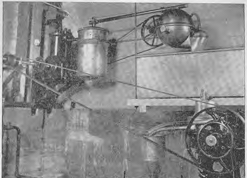
Fig. 4.—Separator-room for cream-supply dairy, showing vacuum pump on wall, vacuum tank close to pump, suspended milk vat and hopper of skim-milk pump. Base of 4 ft. of concrete under walls.
