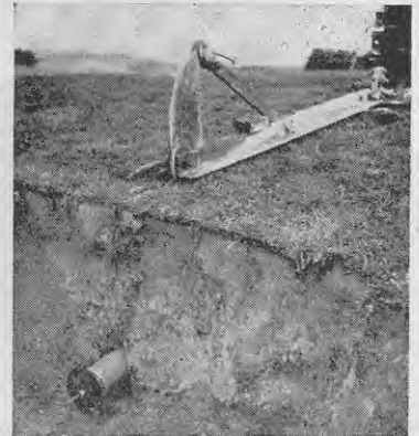
Fig. 3.—Although this bank was rather dry, a 2½ in. pipe (outside about 4 in.) is pulled in quite readily behind a 3 in. plug.
