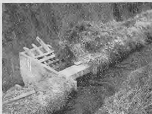
Fig. 17.—The intake and screen, showing the surplus water lead off to the right in this scheme.
