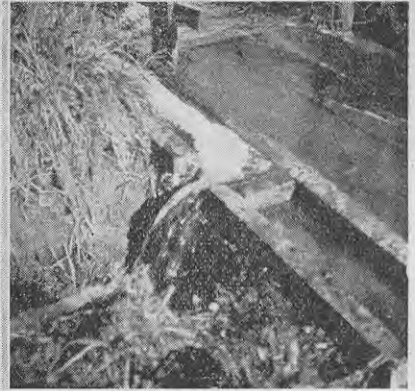
A block in the drain to the sump diverts rain or other unwanted water from the sump.
