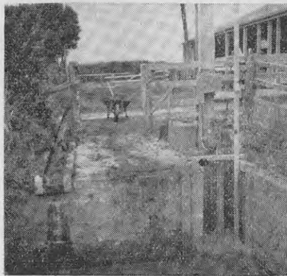
Fig. 5.—An electric pump is used here to lift the manure from the sump to the tank.
