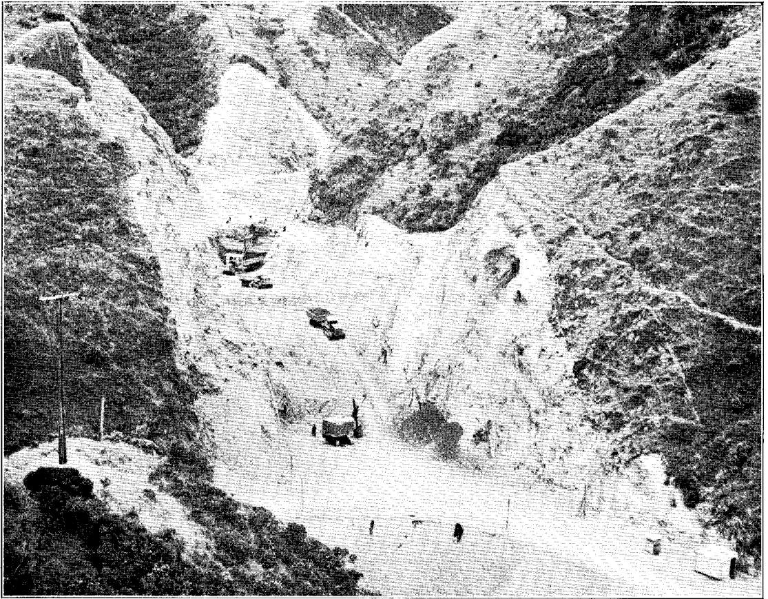
VIEW OF THE MAIN CUTTING LOOKING TOWARDS JOHNSONVILLE. FINAL ALIGNMENT OF THIS SECTION IS ON A 15-CHAIN-RADIUS CURVE. BATTERS ON LEFT WILL BE 145 FT. AND 160 FT.
