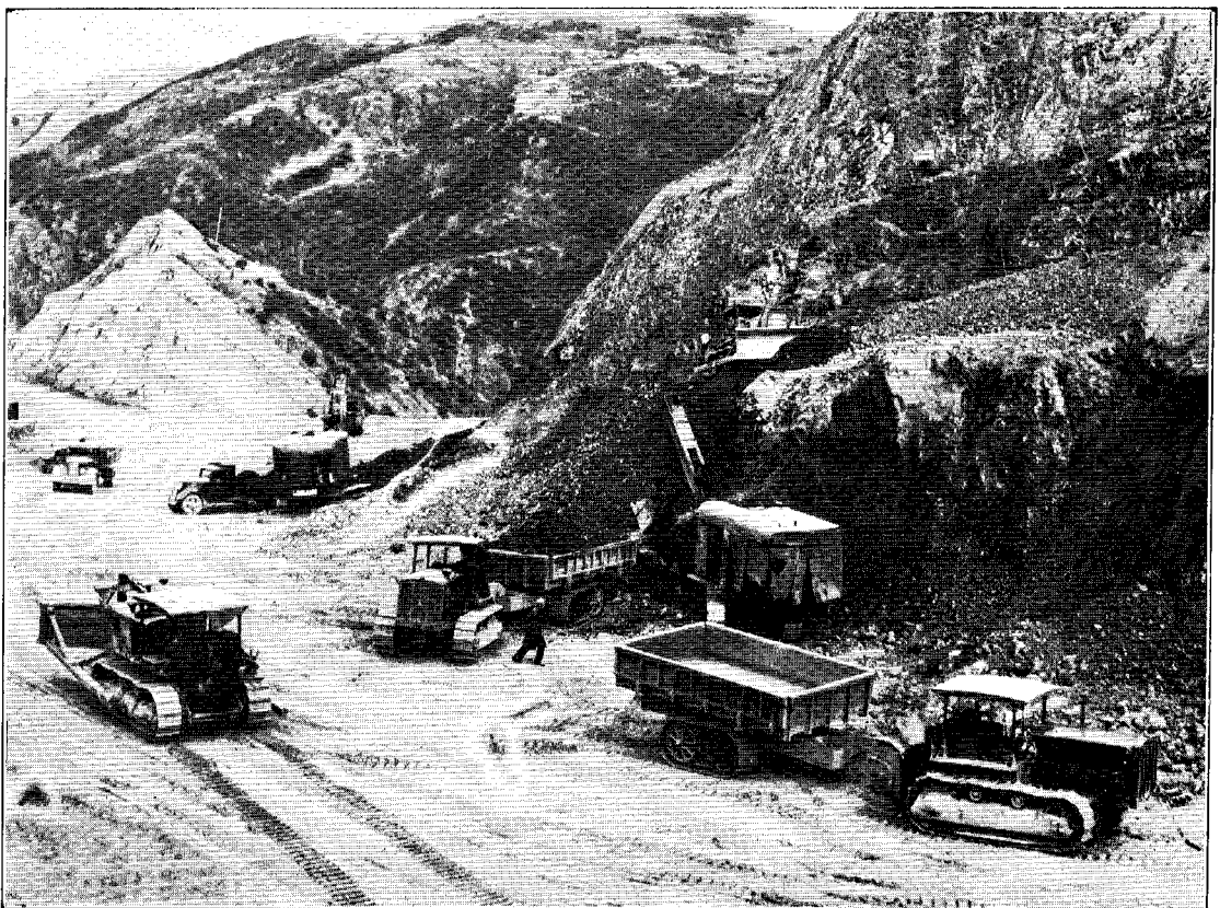
EXCAVATING AND HAULING EQUIPMENT IN OPERATION. NGAHAURANGA GORGE ROAD. WELLINGTON - TAWA FLAT MAIN HIGHWAY.
