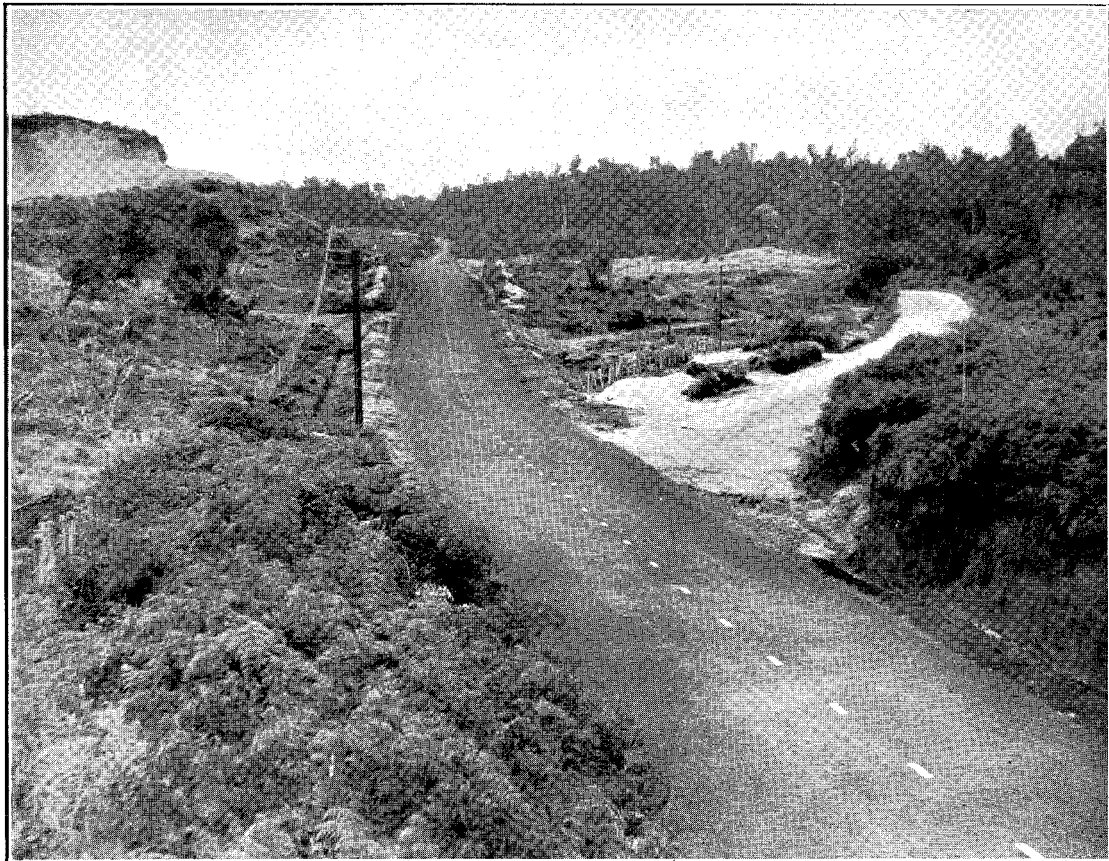
RE-ALIGNMENT AND SEALING ON NGONGOTAHA—MAMAKU BUSH SECTION. HAMILTON—ROTORUA MAIN HIGHWAY, ROTORUA COUNTY DIVISION. 1—Main Highways.
