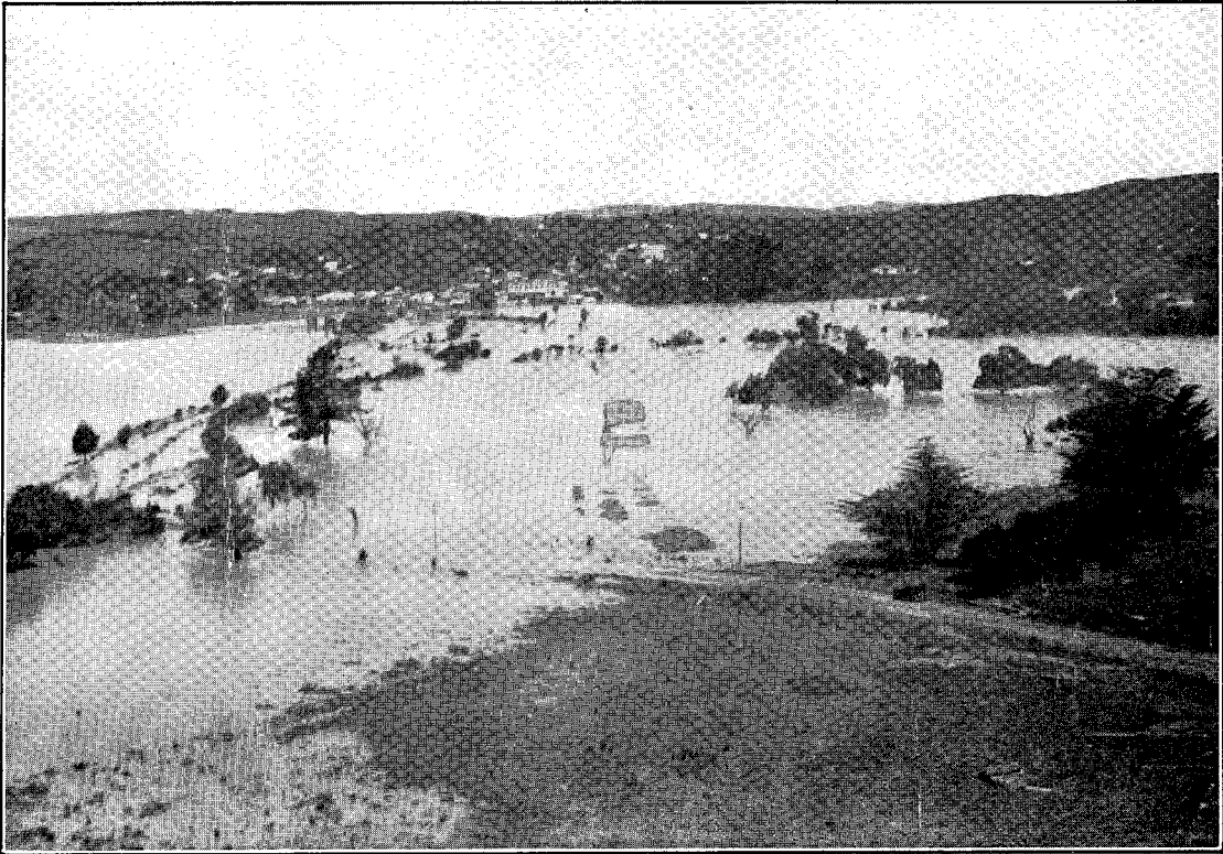
RAISING ROADWAY AT KAWAKAWA TOWNSHIP ABOVE FLOOD-LEVEL ON NEW ALIGNMENT: NEW ALIGNMENT APPEARING IN CENTRE, OLD ROUTE ON LEFT. LAKE OMAPERE—MAUNGATUROTO VIA WHANGAREI MAIN HIGHWAY.
