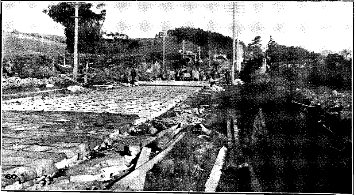
AUCKLAND-WELLINGTON (VIA TARANAKI) MAIN HIGHWAY, MOUNT WELLINGTON SECTION: CONCRETE PAVING IN PROGRESS.
